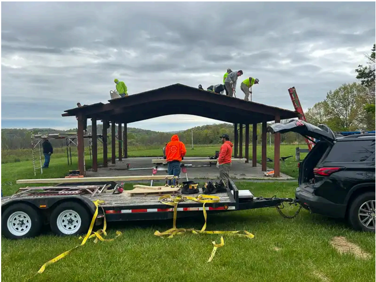
Union volunteers work to repair Vista Pavilion, a 44-by-30 foot shelter located at Blue Marsh Lake's Dry Brooks Day Use Area.
